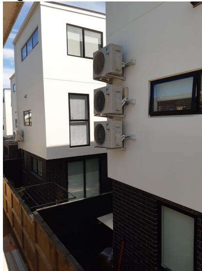
Figure 1: Three external air conditioning units attached to terraced house
