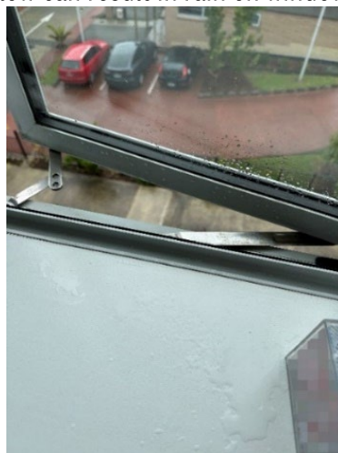
Figure 23: Windows kept open for airflow can result in rain on windowsill
