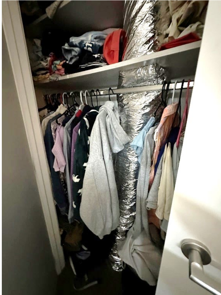
Figure 16: Air conditioning duct in wardrobe
