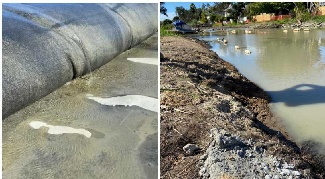
Figure 12. Left: Clear leachate seeping (outlet) from geobags after flocculation. Right: dredging in action (top left) with excavated material containing shells in the foreground.
