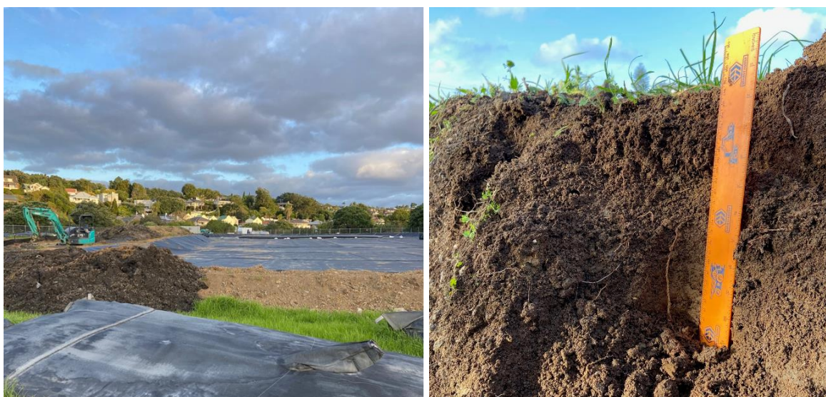
Figure 13. Left: a filled geobag in front of a bund made with natural soil (lighter brown on right) and excavated sediment (darker brown on left). Behind the bund, a black plastic liner is ready for placement of large geobags to be filled with sediment, allowing for the discharge of leachate back to the stream. Right: the soil on the bund is well aerated and has a favourable crumb texture that together allow grass roots to extend to 30 cm depth (the height of the orange ruler).
