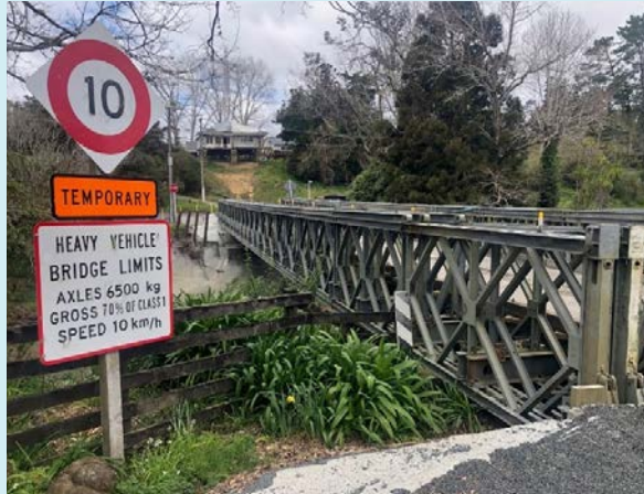
Mill Flat Road bridge washout (left) and repaired bridge (right)
