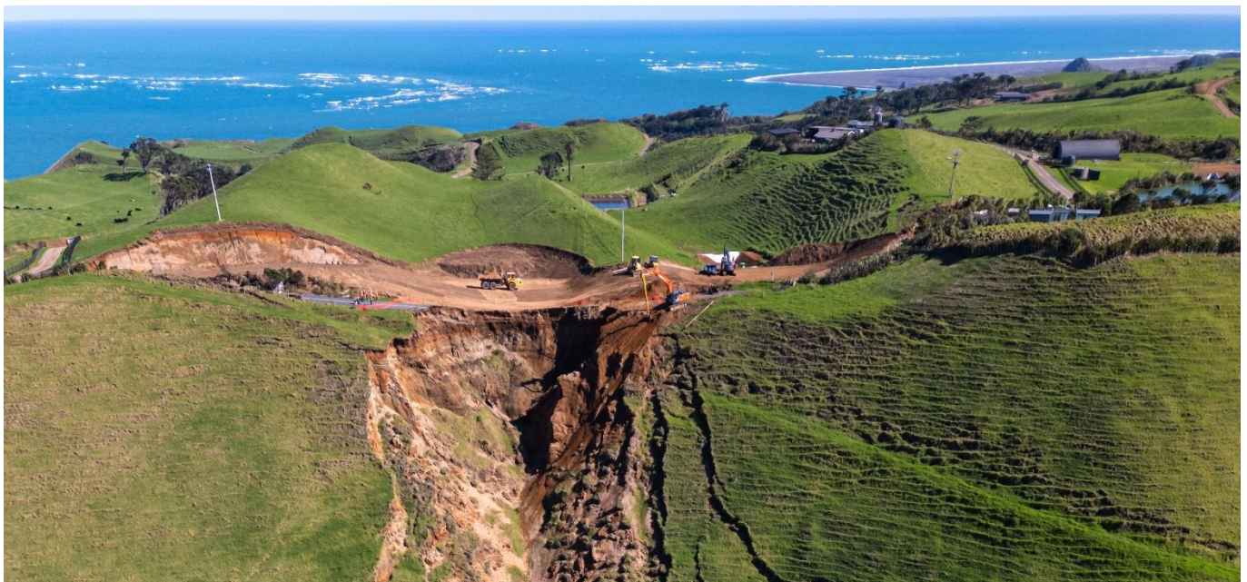
Figure 5. Slip on Manukau Heads Road Source: Auckland Transport
