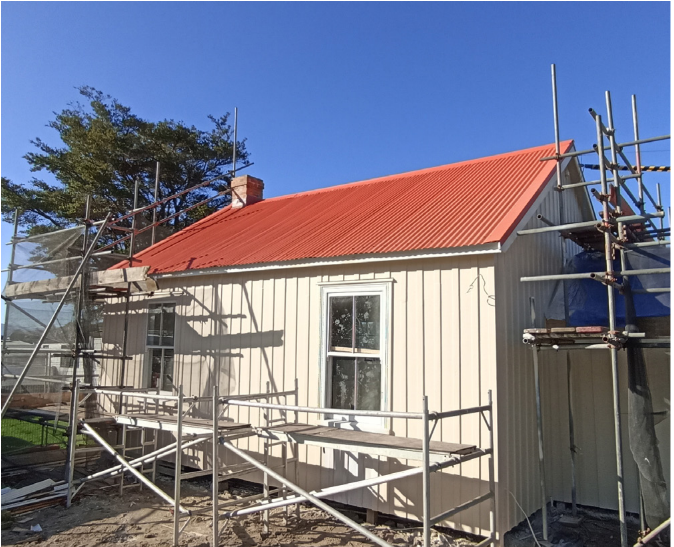
Image: Restoration of the former Sandspit School, Sandspit. Built in the 1880s. © Richard Bland (Heritage Unit, Auckland Council, 2024)
