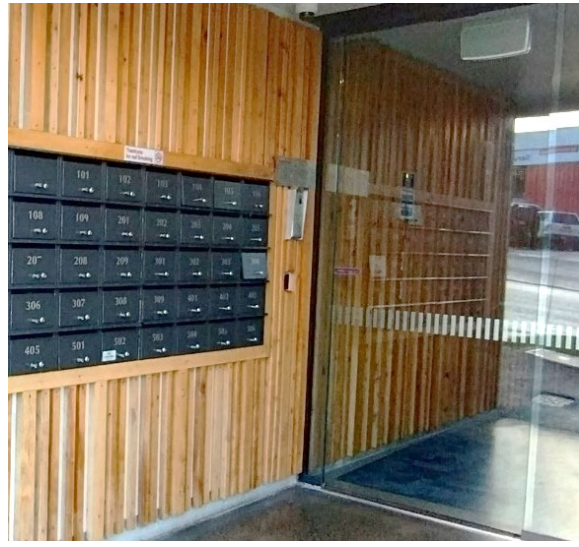
Figure 61: Intercom and swipe card access into an apartment building
