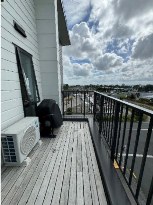
Figure 35: Access to apartment balcony only possible via bedroom
