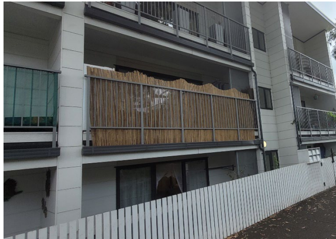
Figure 10: Outdoor living space and primary outlook from living space overlooking the street with additional screening added to balcony balustrade
