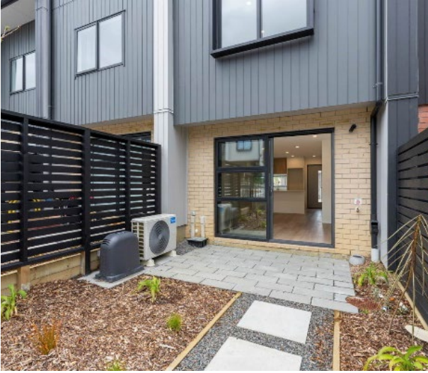
Figure 13: External heat pump unit, pipes and water tank pump in outdoor living space
