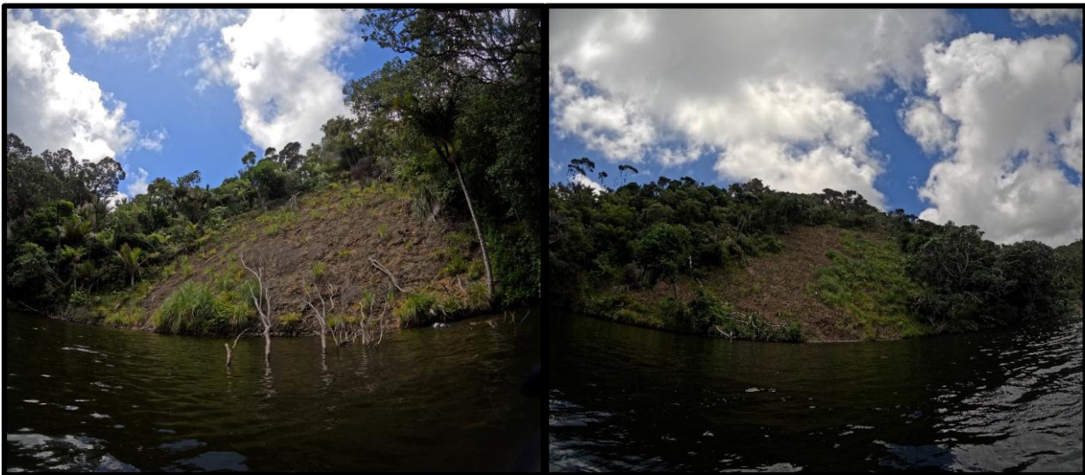
Photo plate 24: Cyclone induced land slips.
